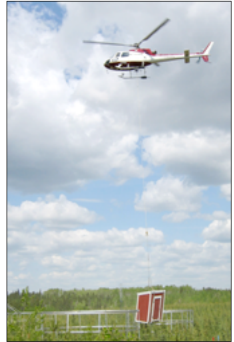
Many of the materials used to build the aluminum frame structures were lifted by helicopter to the research site near Thompson, Manitoba.
